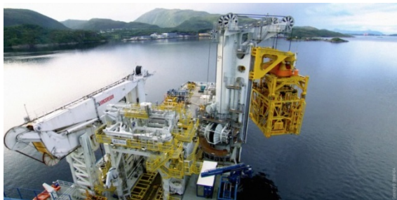
The installation of the compression modules on the Åsgard field - © Statoil ASA
